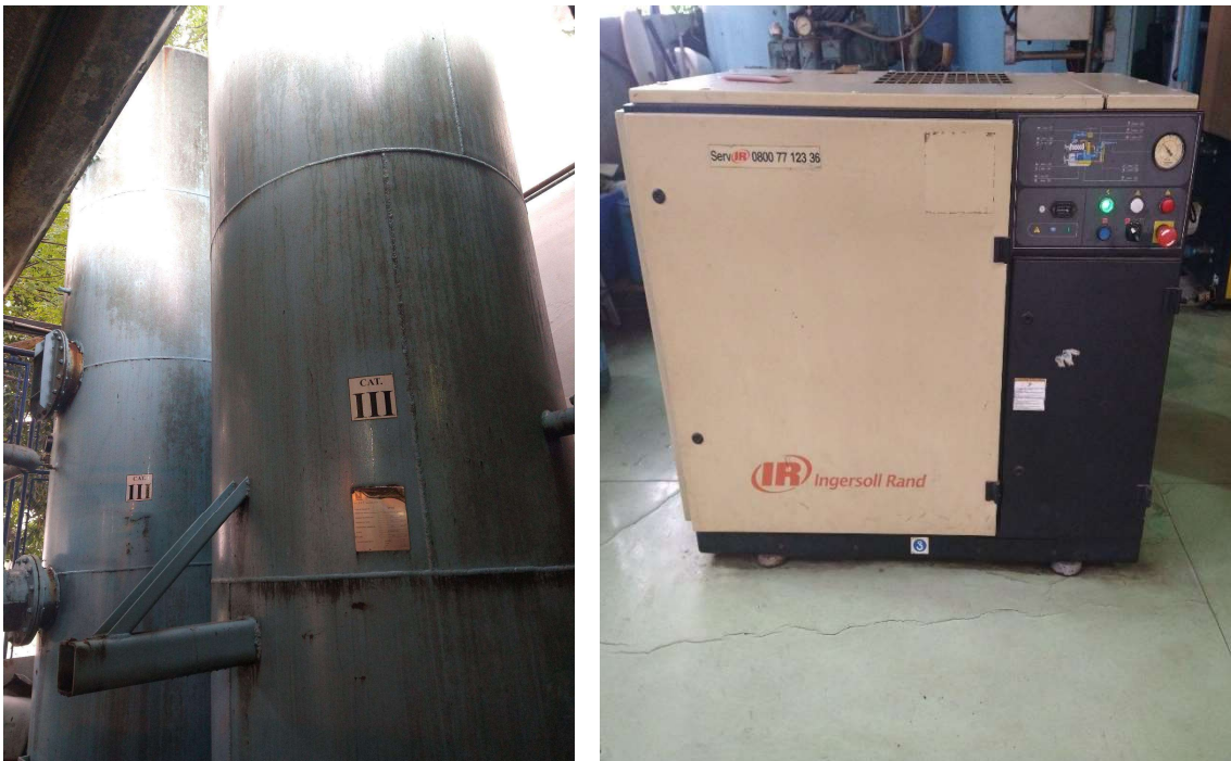
Figure 14: Set of compressed air tanks and compressor
