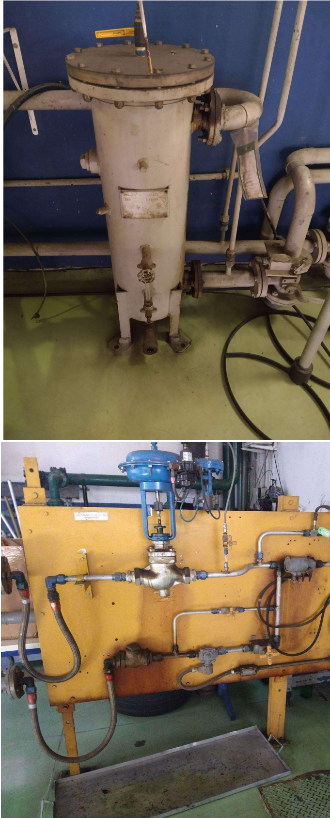
Figure 13: Filter and Fuel Control System
