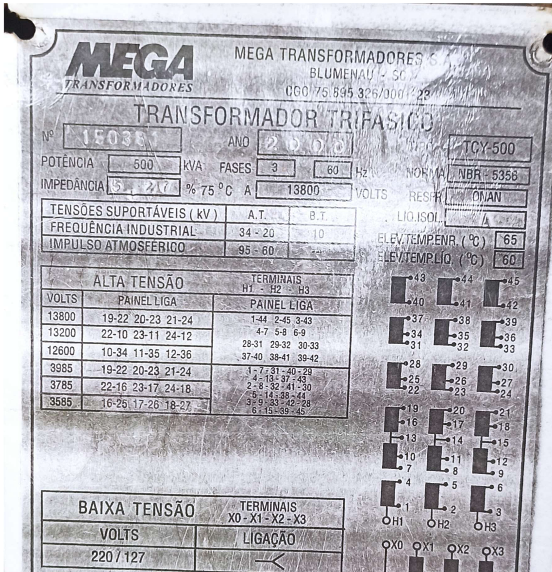
Figure 6: Substation electrical transformer specifications
