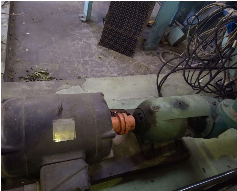
Figure 20: Motor-pump for the fire-fighting system
