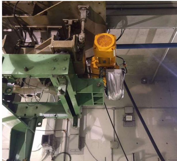
Figure 18: System operated by electric hoists
