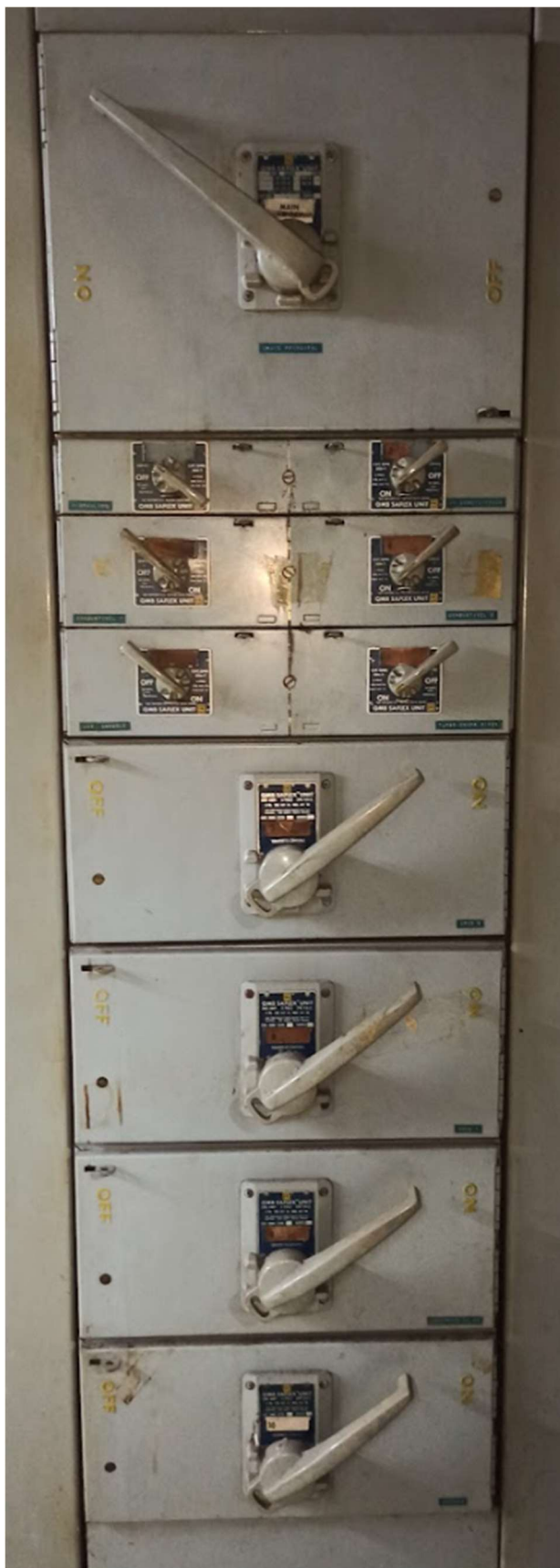
Figure 10: Views of the General Electrical Panel 5
