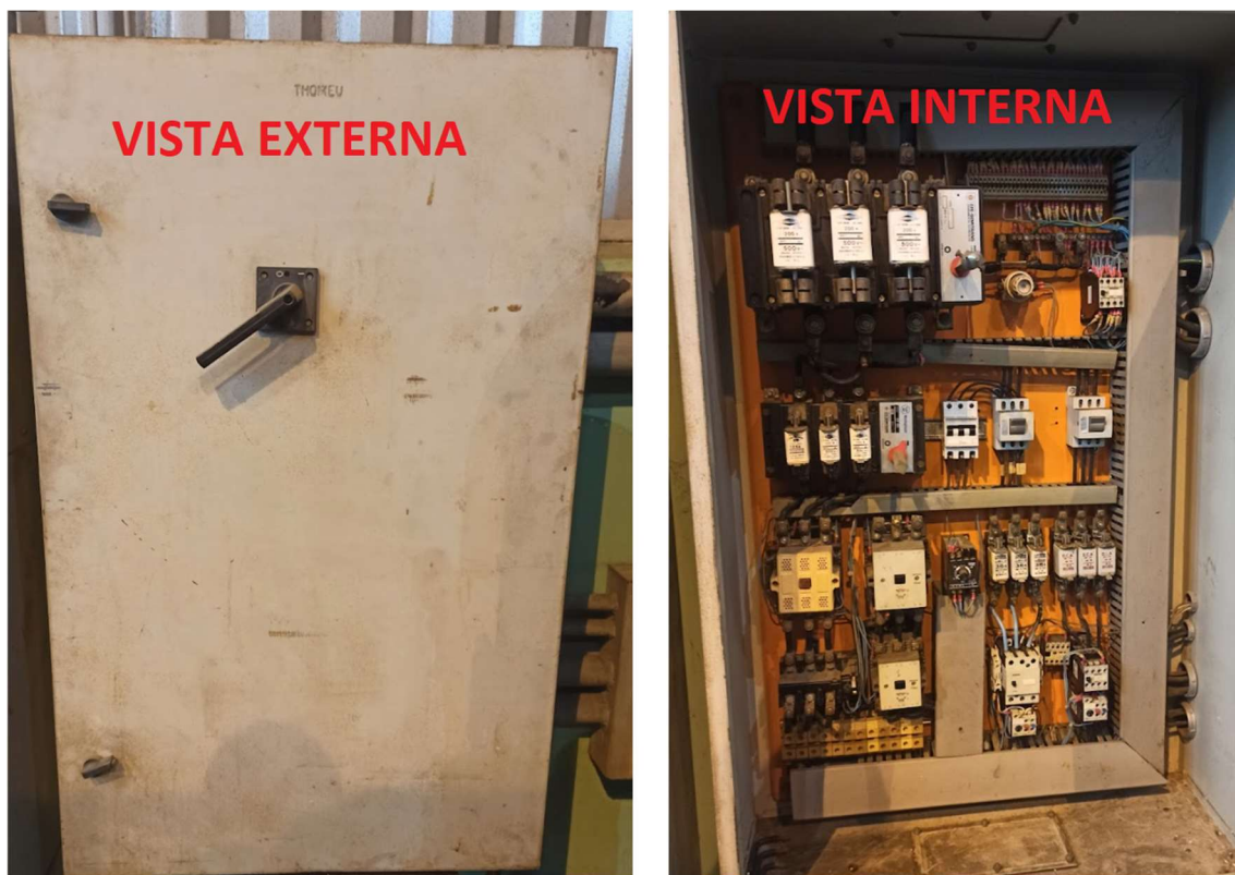
Figure 9(b): Internal and external views of the General Electrical Panel 4
