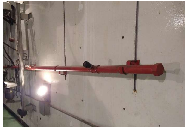
Figure 19: Test cell with the positioning of fire extinguishers
