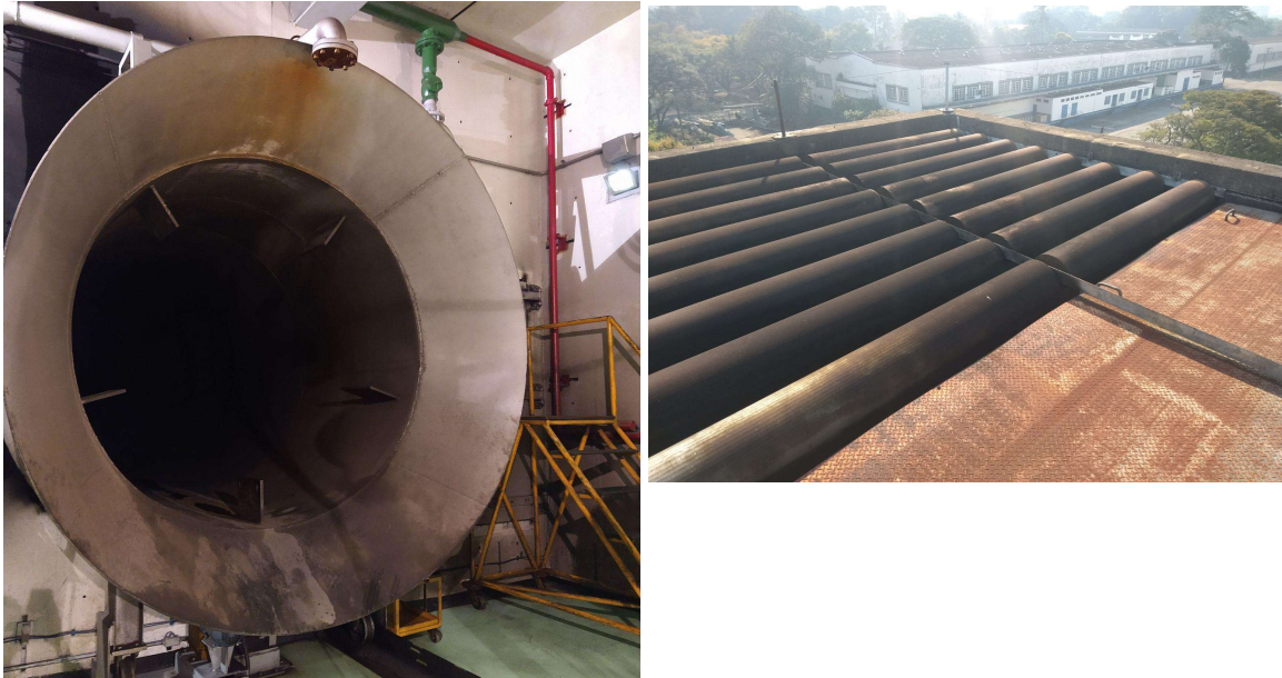
Figure 4: Exhaust gas collection duct with the cooling sprinkler (on the left) and exhaust tower dampers (on the right)
