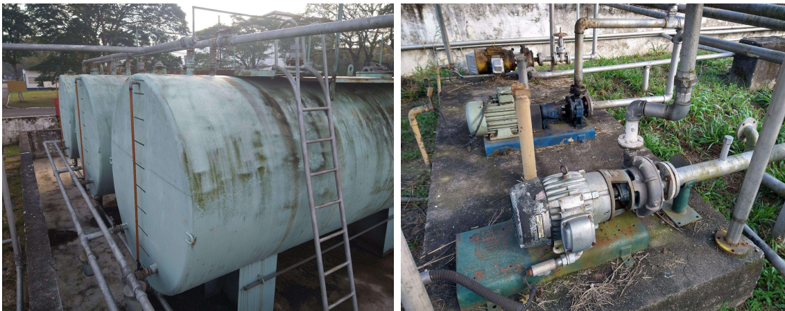
Figure 12: Storage Tanks and Motor Pump Set
